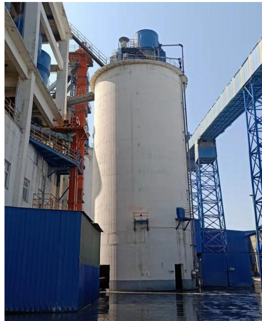
粉煤灰仓密闭储存
